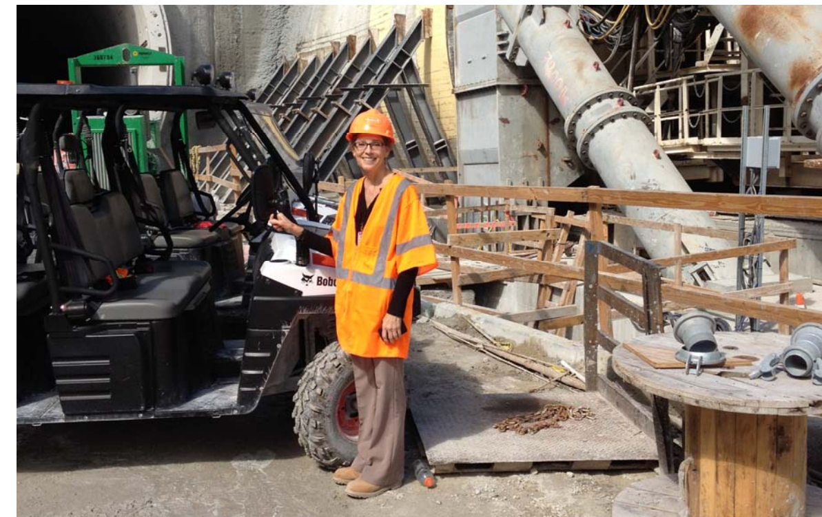
Suzanne standing in front of the tunnel boring machine used to drill the Port Miami Tunnel. "I represented one of the insurance companies during construction and I made about four site visits, which was quite a treat for me."
